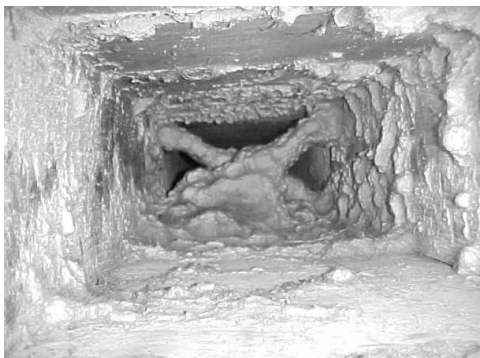
A very contaminated duct.
